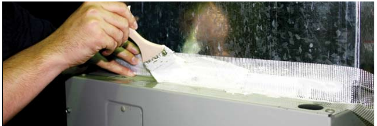
Use mastic and fiberglass mesh tape to connect plenum to air handler
