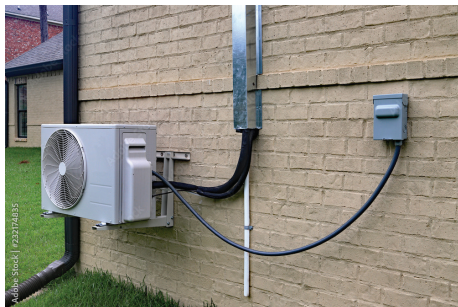
Mini-split heating and cooling systems offer an affordable alternative to less-efficient air-source heat pumps.
