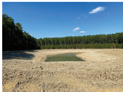
Camp Cale was recently awarded an ACT grant to help with construction of a fishing pond.
