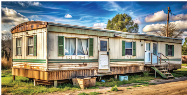
With an investment of time and money, older manufactured homes can be made significantly more energy efficient.
