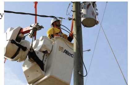
Albemarle EMC Apprentice Lineman Drake Trueblood uses line guards, rubber gloves and sleeves, a helmet and safety glasses to safely work on a transformer.
